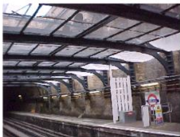
Compression struts requiring strengthening
