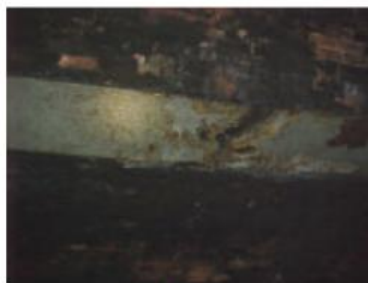
Cast iron beams requiring strengthening
