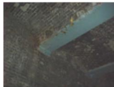
Tunnel roof requiring strengthening
